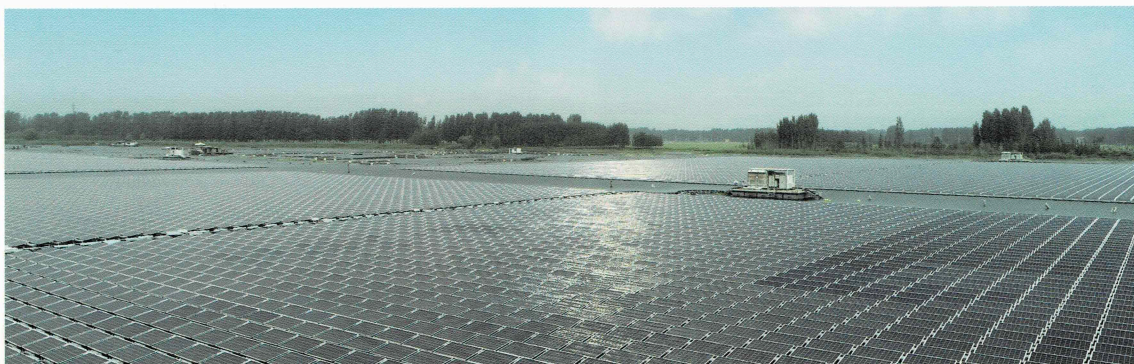
Weishan Jining • China Installed capacity : 100MW
